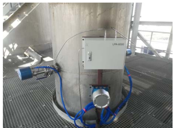
Example of Field Installation
