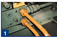
place of installation
